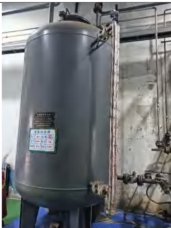
硝基苯焦油废液罐
